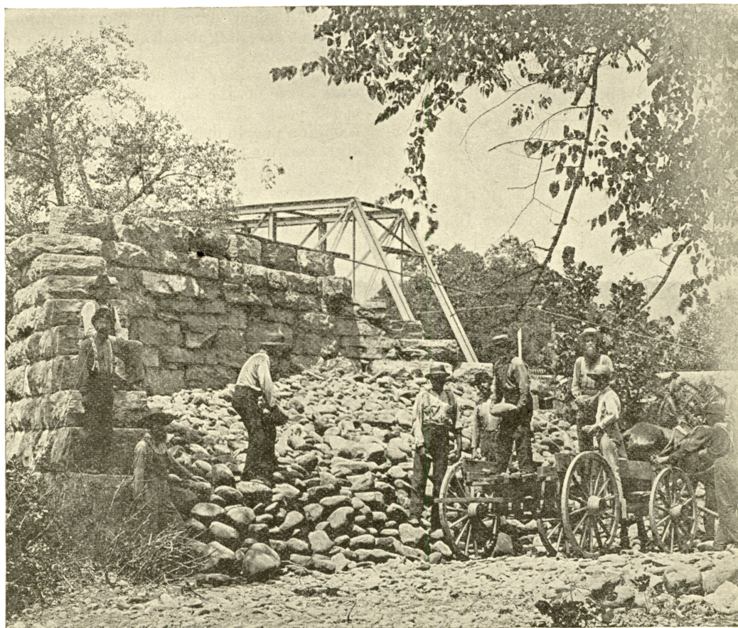
ENFORCING "LAW" IN THE UNITED STATES.—Seventh-day Adventists Compelled to Work on the Public Roads in Tennessee.
